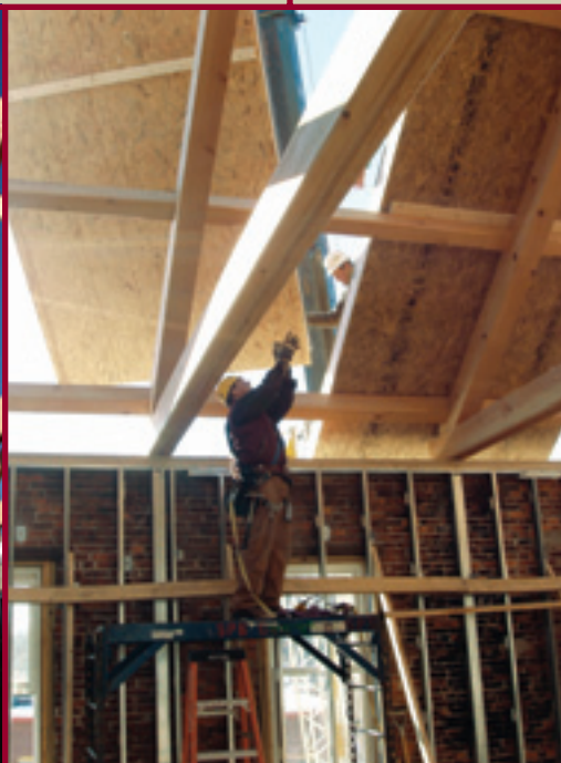
Workers guide an 8-foot by 24-foot roof panel into position on purlins.
