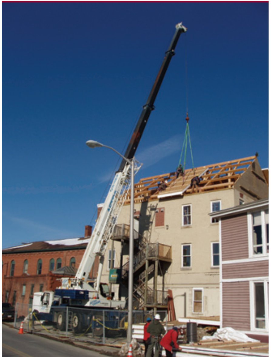
Benson Woodworking crew employs a Krupp crane provided by Astro Crane to position roof panels for Museum of Russian Icons in Clinton, Mass.
