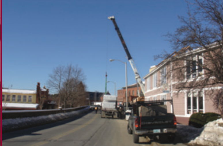
Police detail closes off one-lane of narrow section of Route 62 as crane unloads pallet of prefabricated roof panels.
