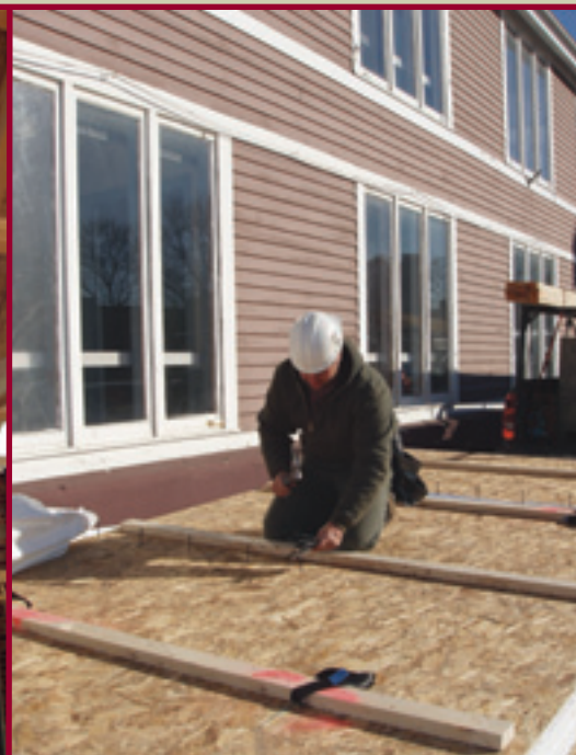
Duane Beiler pre-installs extra-long screws that will later be driven to hold panels to purlins.
