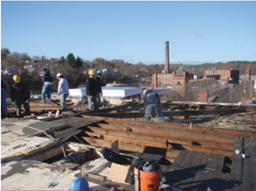
Top left: Murray Brothers Construction workers demolish roof of old mill building being converted into museum.
