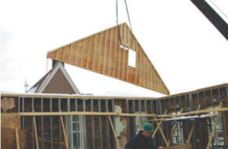
For lack of space, gable end walls were fabricated on third floor, then lowered to alleyway at street level until ready for final positioning.
