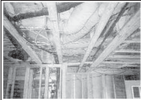
If mechanicals are unplanned, poorly designed, or haphazardly installed, they can get seriously entangled. This makes repairs or upgrades difficult. (photo by Stephen Kendall)
