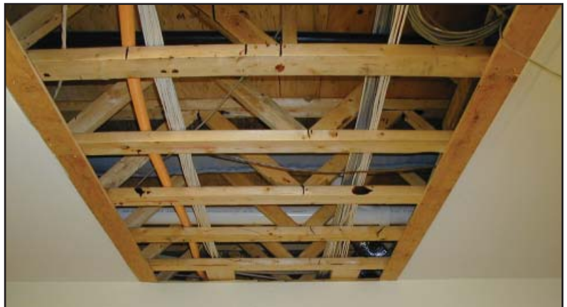
Open webs between the floor and ceiling for electrical, plumbing, and heating ducts make installation and later renovations relatively simple.
